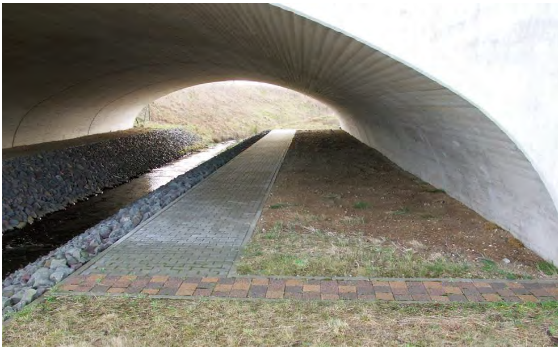
Fig. 23: Poor design of water course passages
